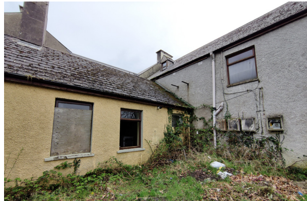
Derelict building and court along Main Street, Creeslough © Arup
